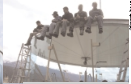
Above: Perrault's team took this photo of construction workers sitting on the café's roof, which is supported by its structural laminated glass 'walls', as a parody on Frank Lloyd Wright's 1920s photo of workers sitting atop one of his first reinforced steel structures. The message from the architect in both cases was: "It holds!"
